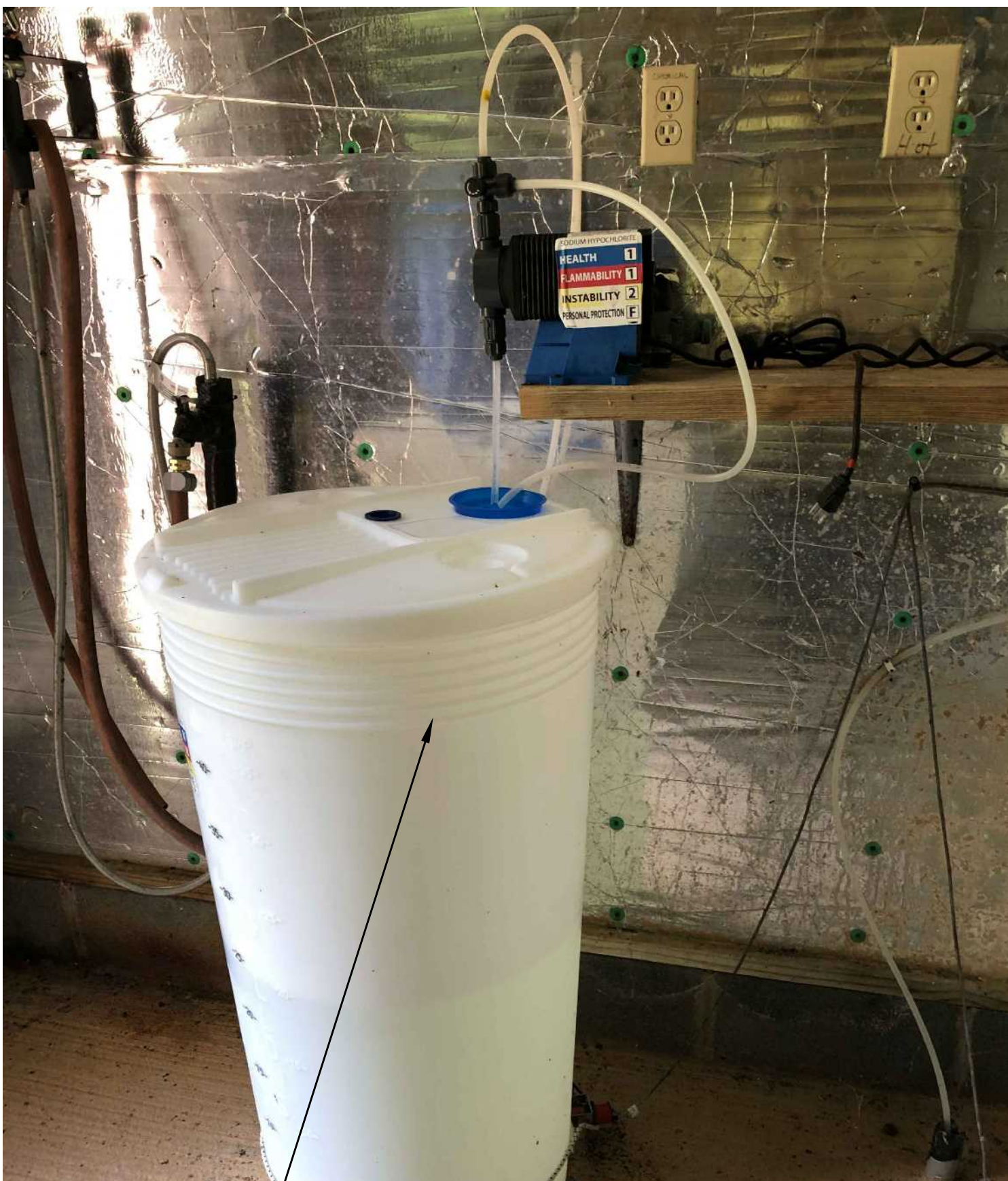
CHEMICAL TANKS AND PUMPS
