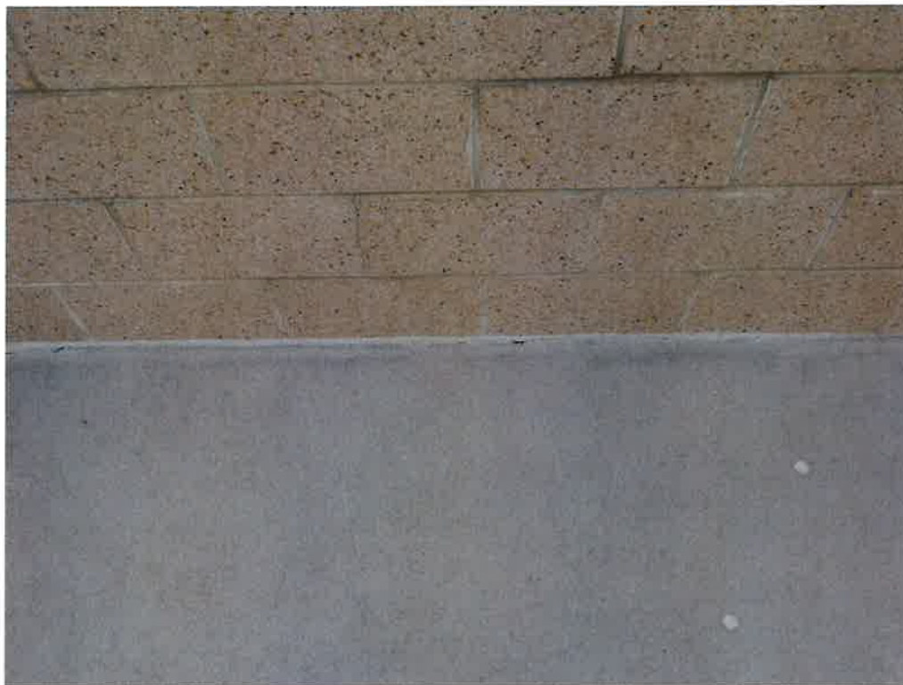
13. Close-Up View of Stitch Pattern in Concourse Area Edge of Elevated Slab / CMU Parapet Wall Joint Caulk/Sealant Lost Adhesion at West Side of the Area.
