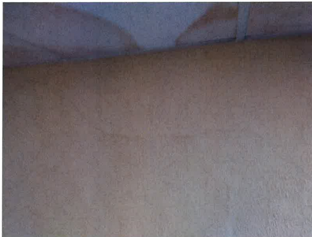
44. Close-Up View of Diagonal Hairline Crack in the Concrete Load Bearing South Wall of the Club House Level Home Team Locker Room.
