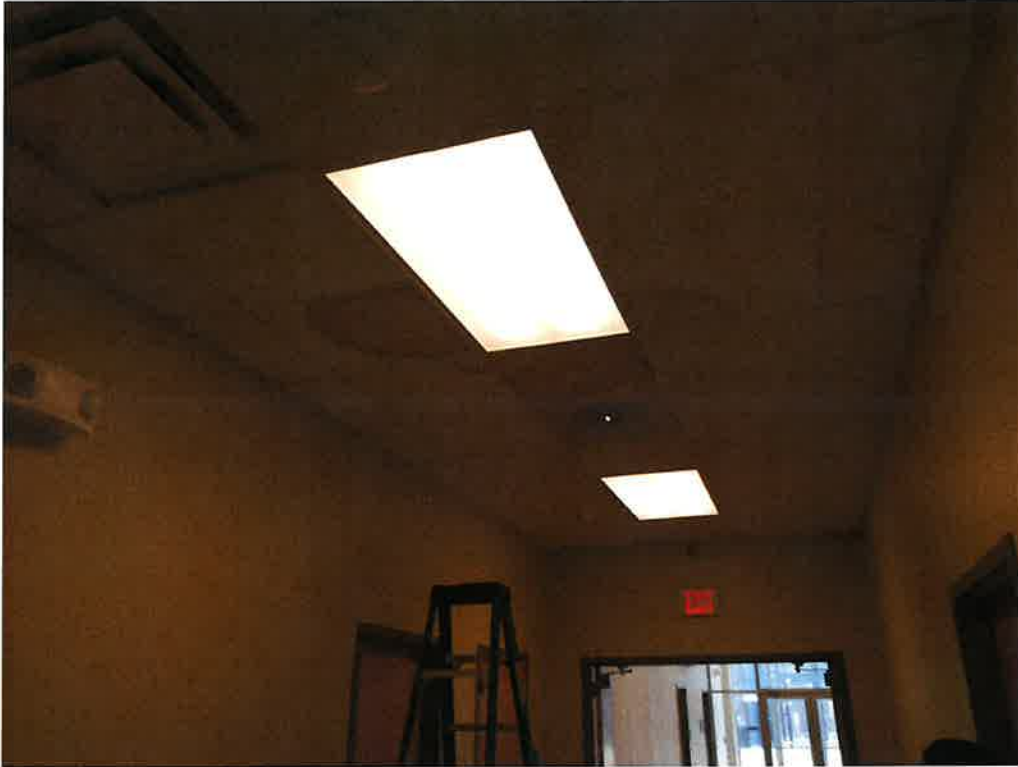
33. View Looking at Water Stained Ceiling Tiles in the Club House Level Corridor.
