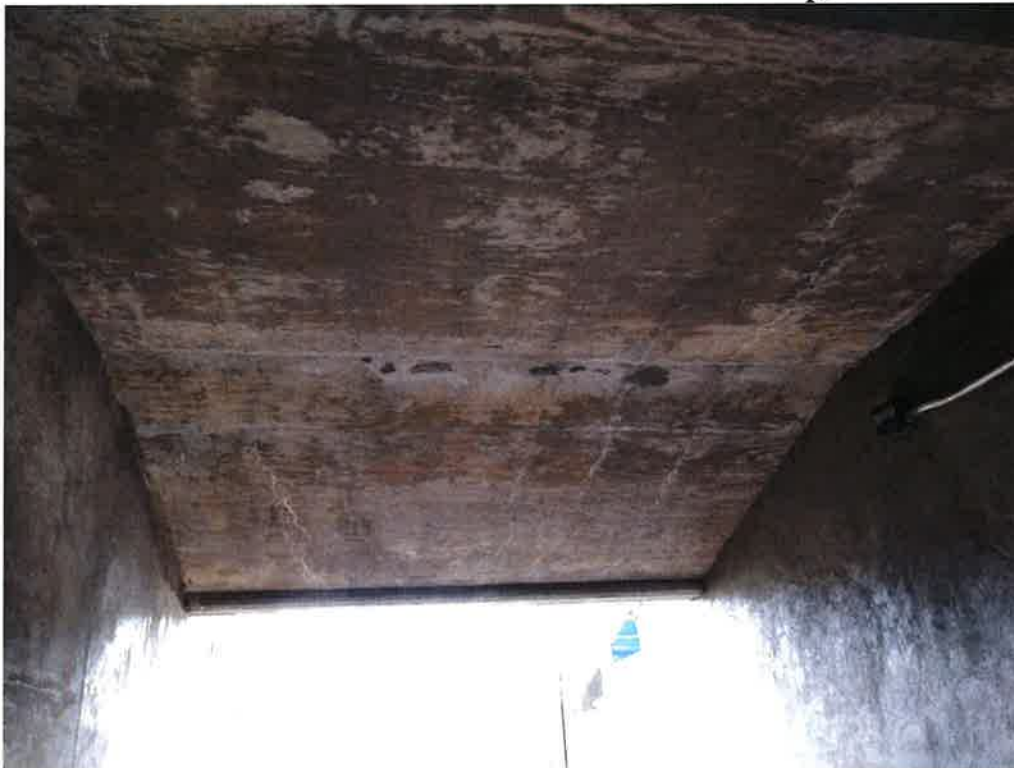
38. View Looking at the Linear Cracks & Possible Efflorescence Leeching from the Cracks in the Exposed Concrete Ceiling of the Home Team Access Ramp.
