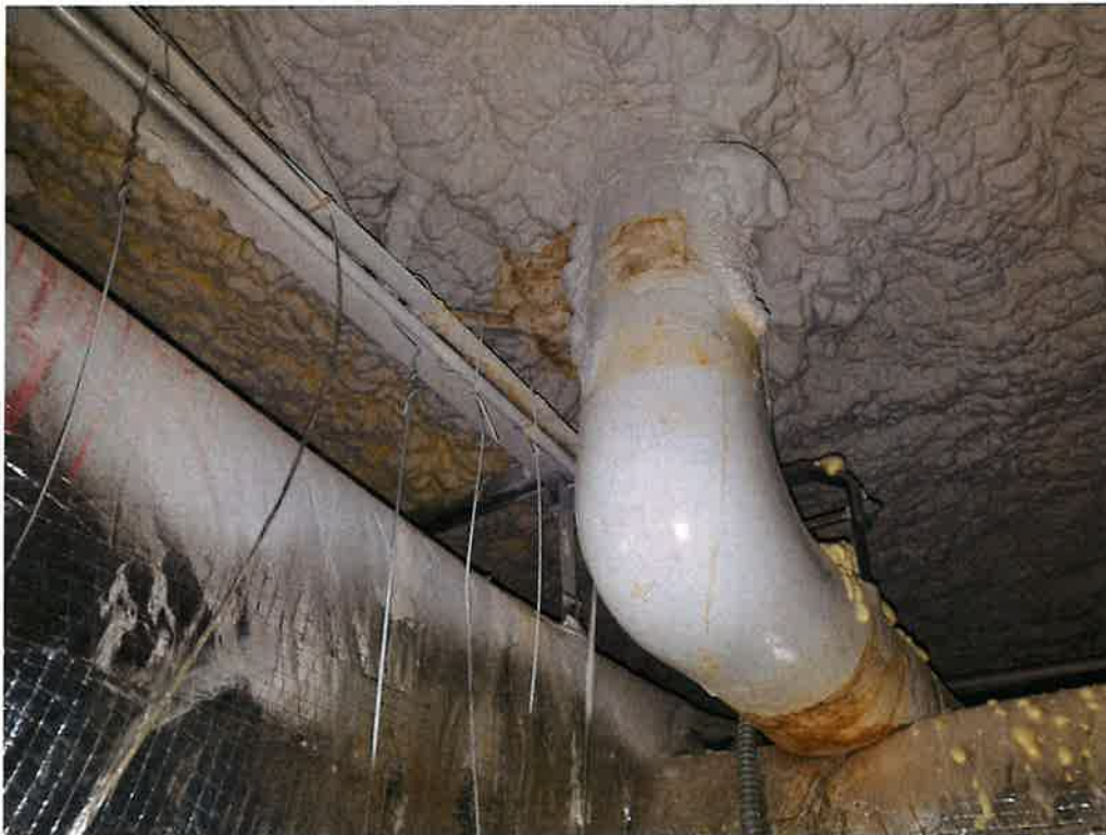
34. View Looking at Club-House Level Water Stains on Insulation Above the Corridor Ceiling Tiles & Appears Adjacent to Concourse Area Storm Drain.
