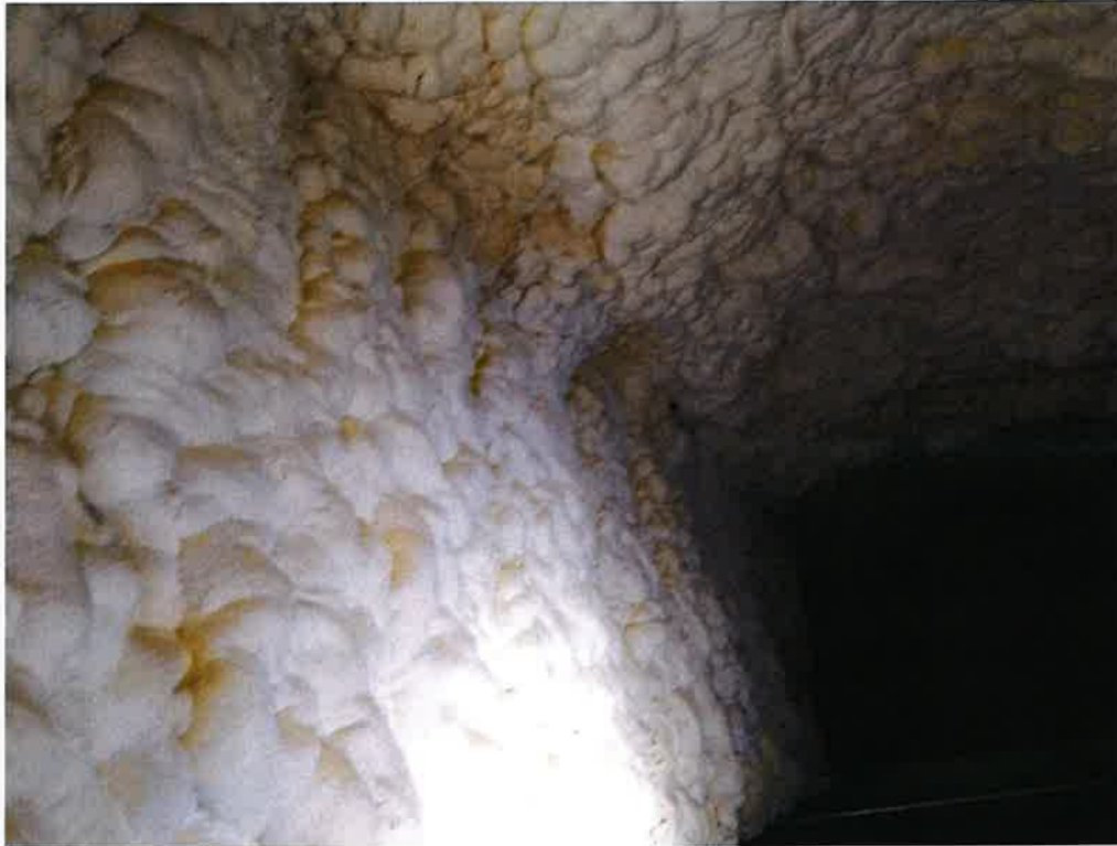
31. Close-Up View Looking at Club-House Level Water Stains on Insulation Below the Concourse Area Elevated Slab.
