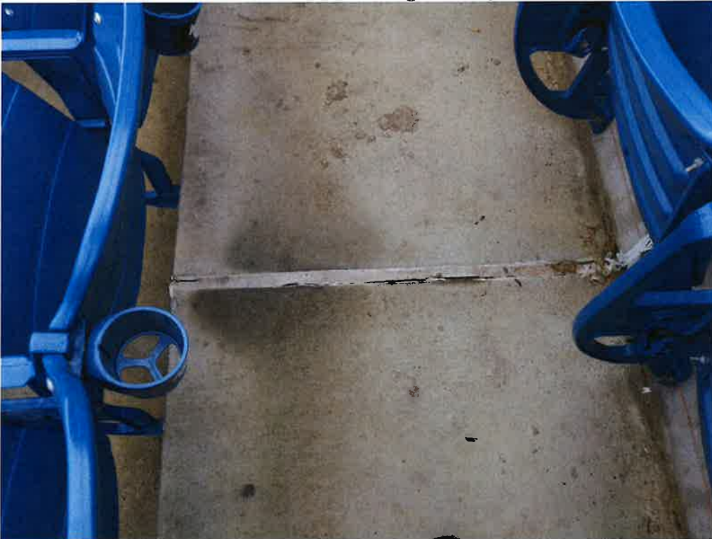
24. Close-Up View of Area in Top Surface of Stadium Seating Slab-On-Grade w/ Stitch Pattern Where Joint Caulk/Sealant Lost Adhesion.
