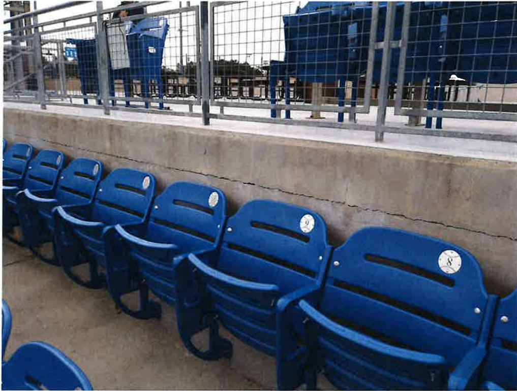
19. View Looking at Stadium Seating Area Horizontal Joint Crack at the Top of Load Bearing Wall / Edge of Concourse Area Elevated Slab (Section 109).
