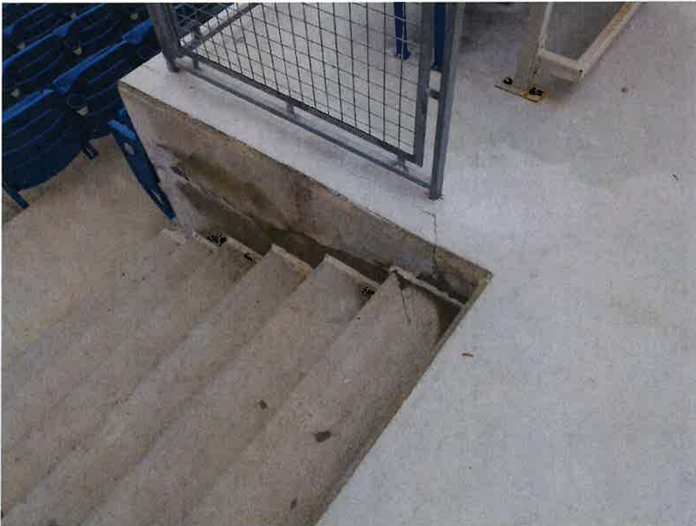
16. View Looking Down at Stadium Seating Area Access Stair / Concourse Area Top Slab Top & Side Surface Cracks Observed at Seating Section 111.
