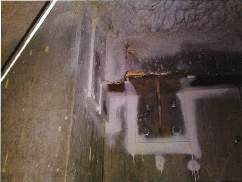
35. View Looking at Club-House Level Water Stains on Insulation Above the Toilet Room 030 Ceiling Tiles.
