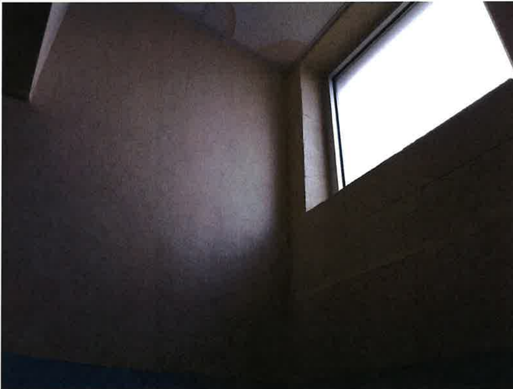
42. View Looking at Water Stained Ceiling Tiles and Interior Paint Peeling from CMU Exterior Wall in the Club House Level Home Team Locker Room.
