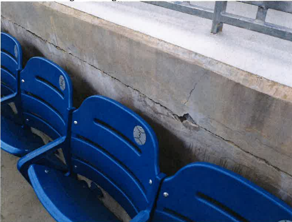
18. View Looking at Stadium Seating Area Crack that has Propagated Up the Face of the Edge of Concourse Area Elevated Slab from the Horizontal Joint Crack.
