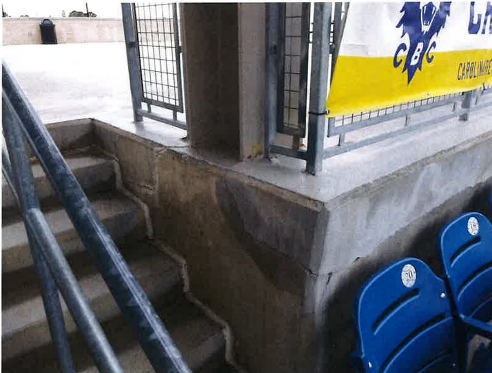
26. View Looking at Stadium Seating Area Horizontal Joint Crack at the Top of Load Bearing Wall / Edge of Concourse Area Elevated Slab at Colum K-4.
