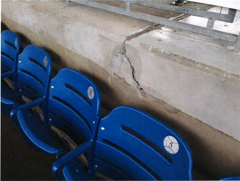
27. View Looking at Stadium Seating Area Where Slab-On-Grade has Spalled at Joint Edge at the Top of Load Bearing Wall at Seating Section 105.
