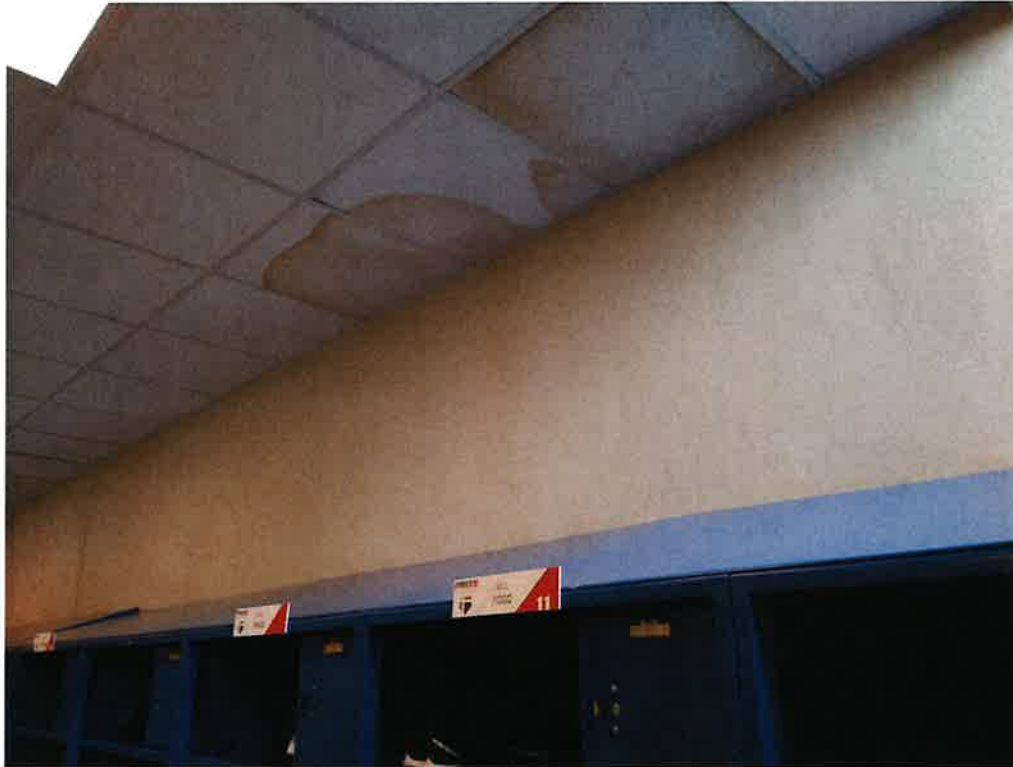
41. View Looking at Diagonal Hairline Crack in the Concrete Load Bearing South Wall of the Club House Level Home Team Locker Room.
