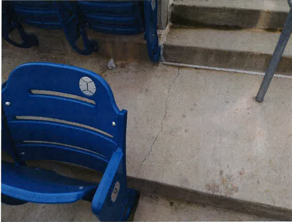
21. Close-Up View of Hairline Crack Observed in the Top Surface of the Stadium Seating Slab-On-Grade.
