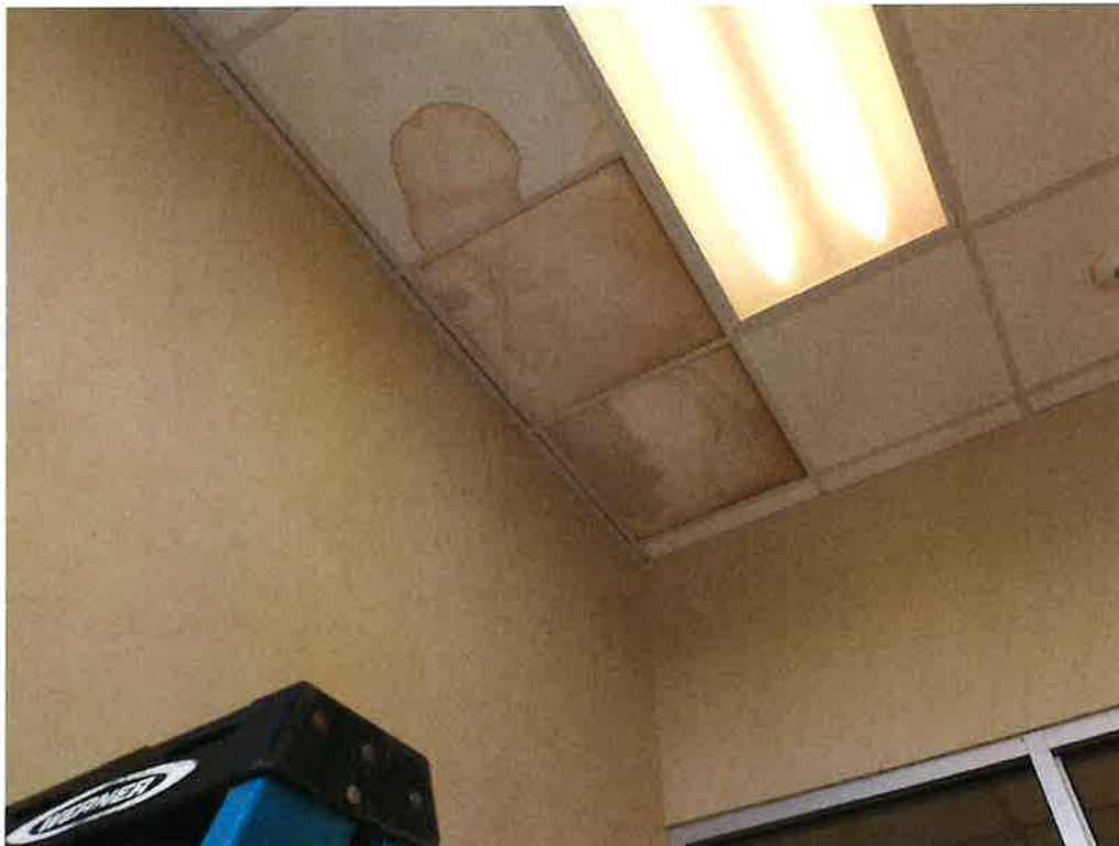
32. View Looking at Water Stained Ceiling Tiles in the Club House Level Entry Vestibule.
