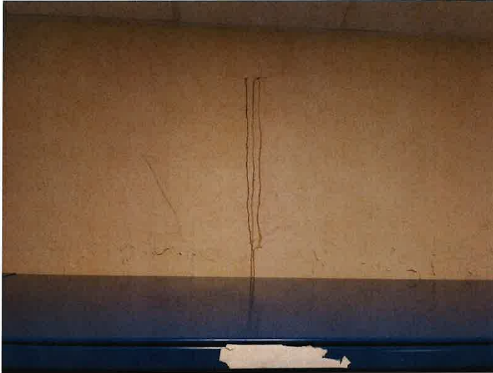
43. View Looking at Crack / Potential Thru Wall Crack in the Concrete South Wall of the Club House Level Home Team Locker Room.
