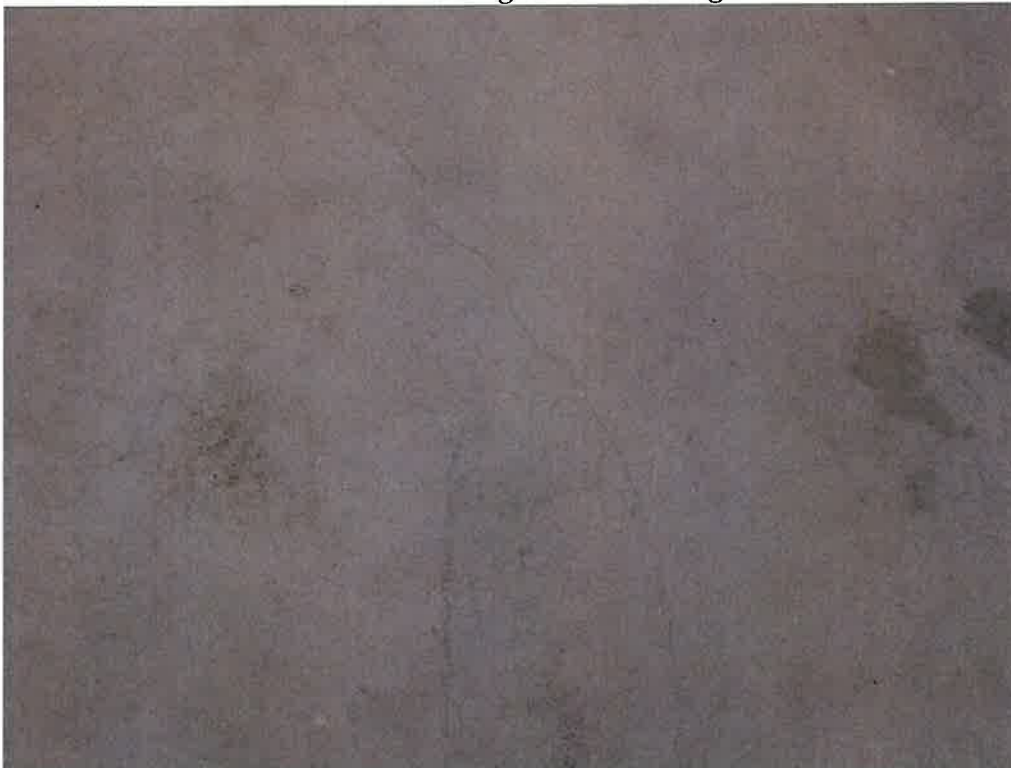
8. Close-Up View Looking at Linear Crack Pattern Observed in the Concourse Area Elevated Slab Assembly's Top Slab.
