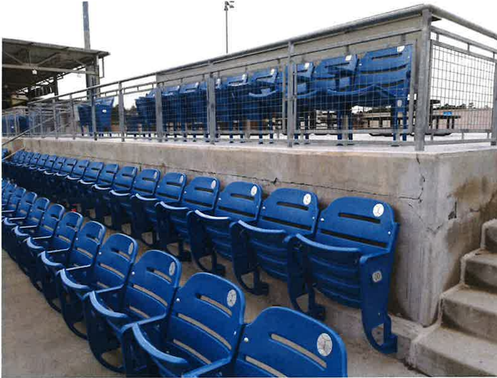
17. View Looking at Stadium Seating Area Horizontal Joint Crack at the Top of Load Bearing Wall / Edge of Concourse Area Elevated Slab (Section 111).
