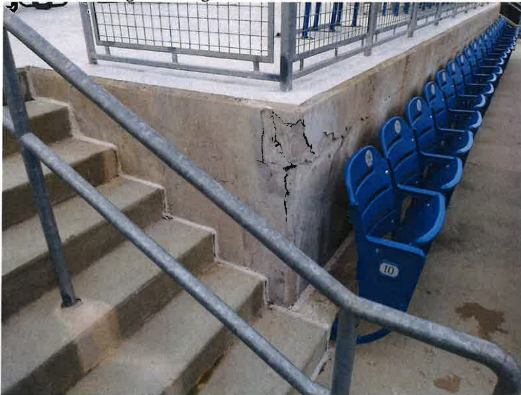
20. View Looking at the Stadium Seating Area Surface Coating Peeling & Delaminating Above/Below the Horizontal Joint Crack (Section 109).
