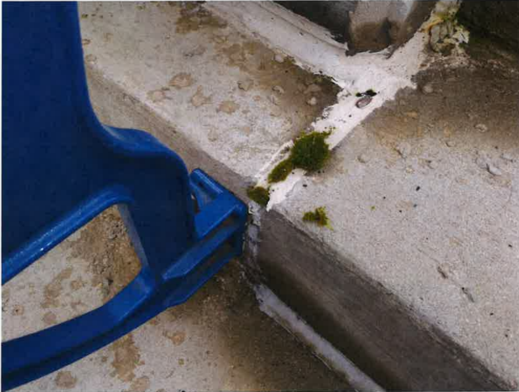
23. Close-Up View of Area in Top Surface of Stadium Seating Slab-On-Grade Where Observed Moss Growing Out of Joint Caulk/Sealant.
