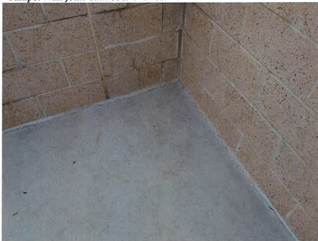
14. Close-Up View of Stitch Pattern in Concourse Area Edge of Elevated Slab / CMU Parapet Wall Joint Caulk/Sealant Lost Adhesion at the Northwest Corner of the Area.
