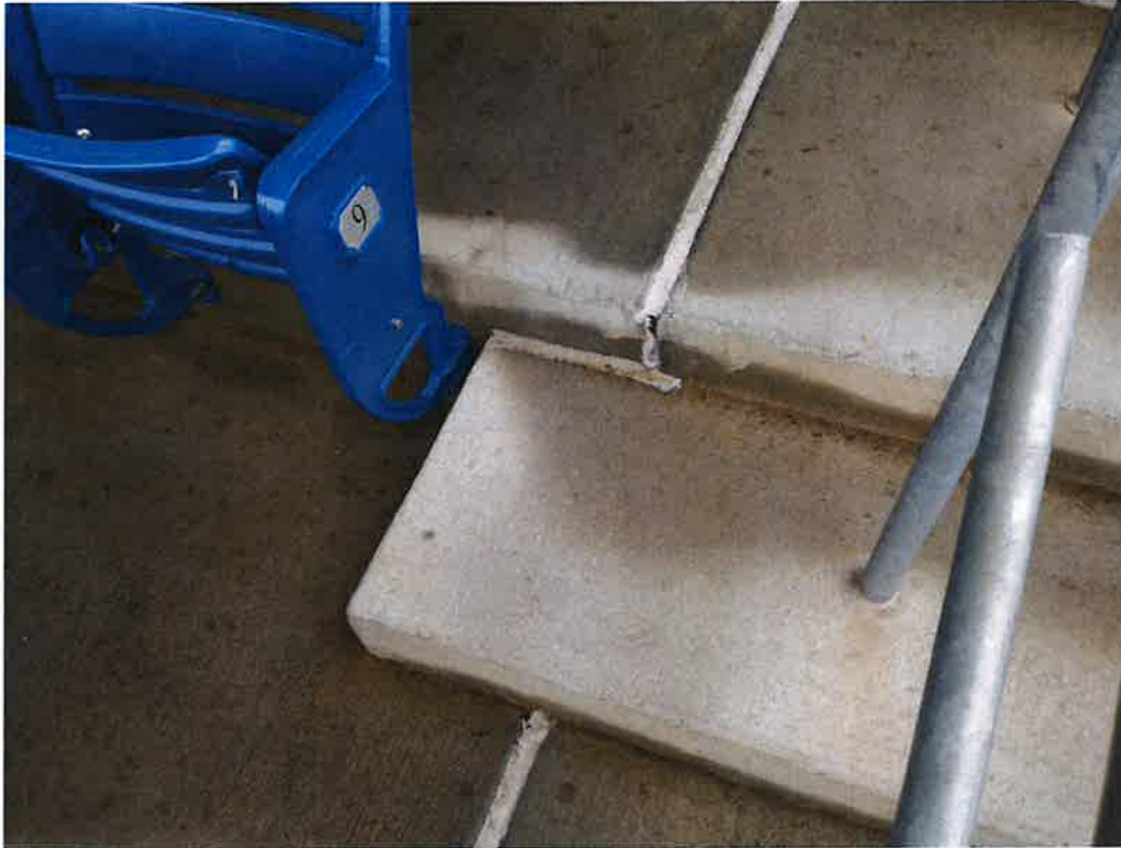
25. Close-Up View of Location Where Stadium Seating Slab-On-Grade Joint Caulk/Sealant Lost Adhesion.
