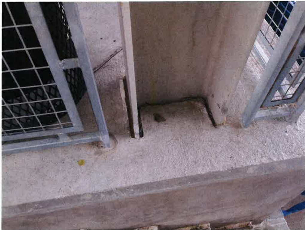
30. Close-Up View of the Expansion Joint that Appears to have Dislodged & Fallen Into Gap Between Steel Column (H-4) & Edge of Concrete.
