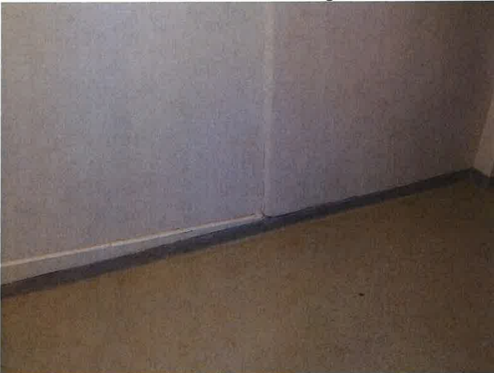
36. View Looking at Vertical Hairline Crack in Base of Wall at Wall Joint in Club House Level Interior Corridor Wall at Corridor to Home Team Field Access.
