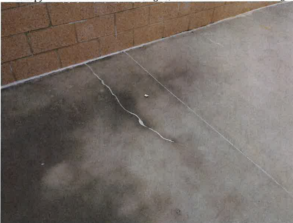
4. Close-Up View of Repaired Linear Crack in Concourse Slab-On-Grade Adjacent to the West Side CMU Parapet Wall.
