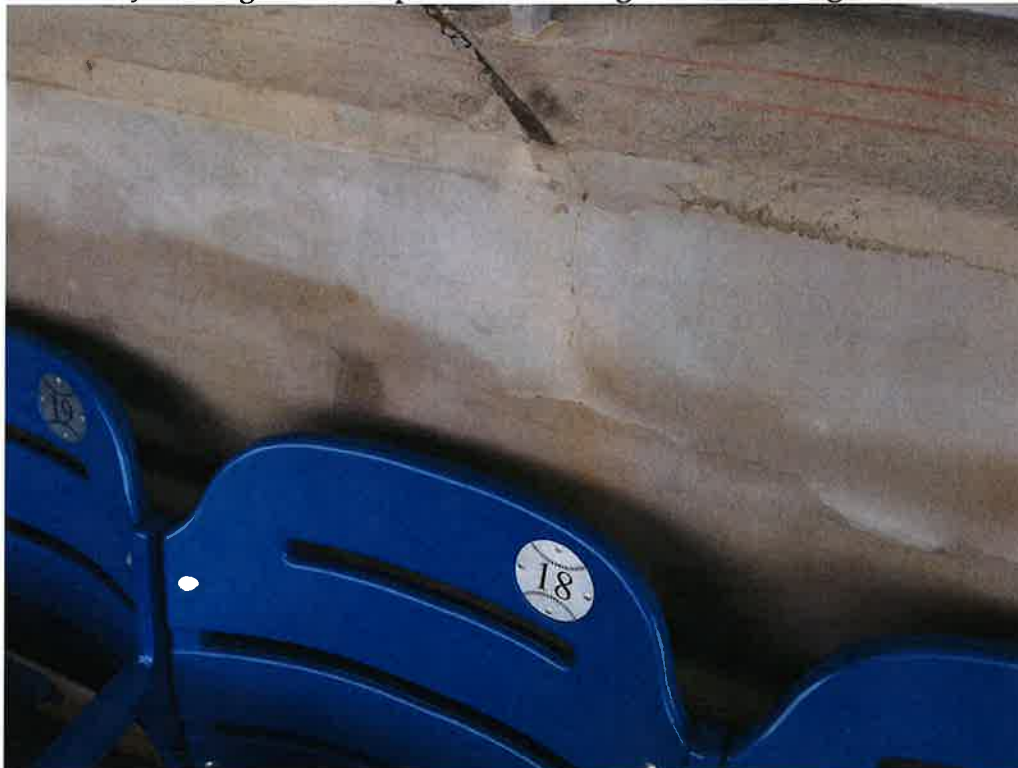
28. View Looking at Stadium Seating Area Where Crack Propagated Down the Face of the Slab-On-Grade at the Column G-4 Isolation Joint.
