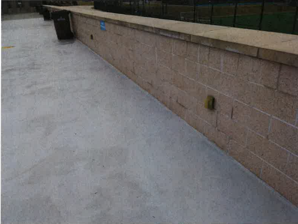
15. View Looking South at the Concourse Area CMU Parapet Wall & the Efflorescence Observed.
