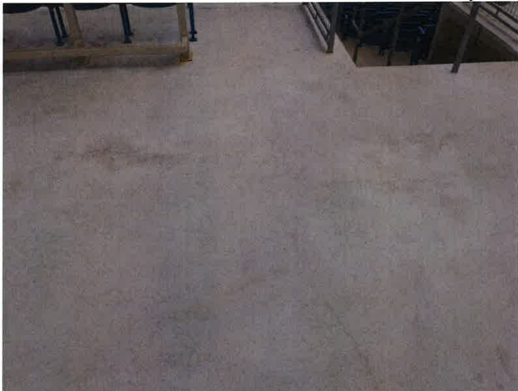
10. Close-Up View Looking at the Linear & Map Crack Patterns In the Concourse Area Elevated Slab Near Access Stair to Stadium Seating Section 107.
