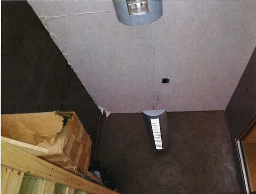
37. View Looking at Paint Peeling from Concrete Ceiling at the Exterior Club House Level Home Team Access Ramp.
