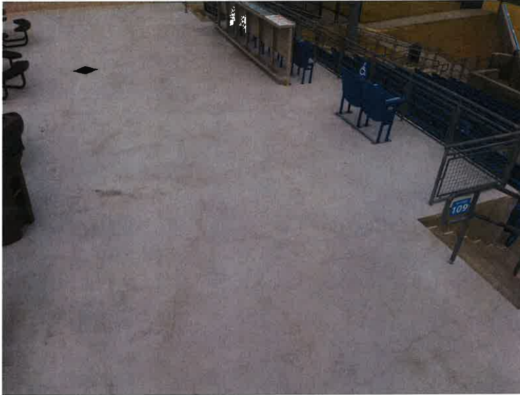
11. View of the Linear & Map Crack Patterns In the Concourse Area Elevated Slab Near Access Stair to Stadium Seating Section 109.
