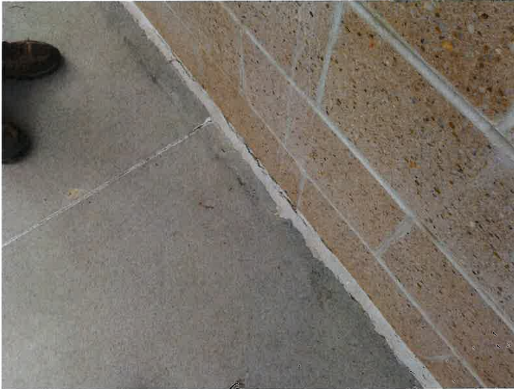
5. Close-Up View of Stitch Pattern in Concourse Area Edge of Slab-On-Grade / CMU Parapet Wall Where Joint Caulk/Sealant Lost Adhesion.
