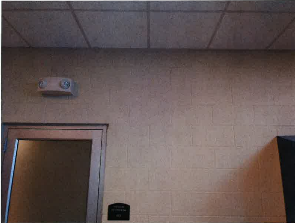
39. View Looking at Step Crack Observed in CMU Load Bearing Partition Wall in the Club House Level Visitor Team Locker Room.
