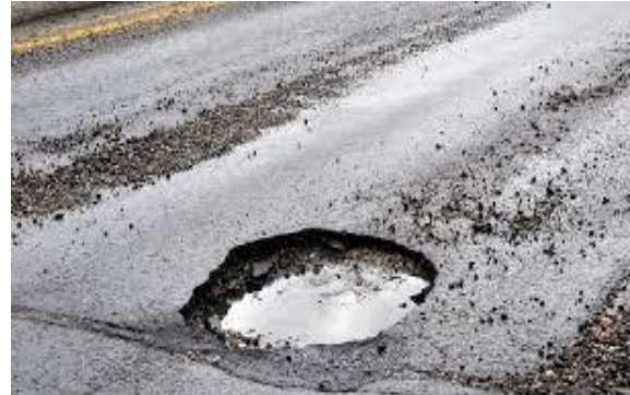
HIGH Severity Pothole
