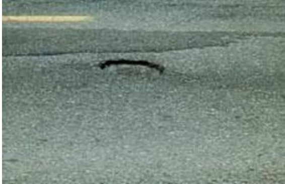
MEDIUM Severity Pothole
