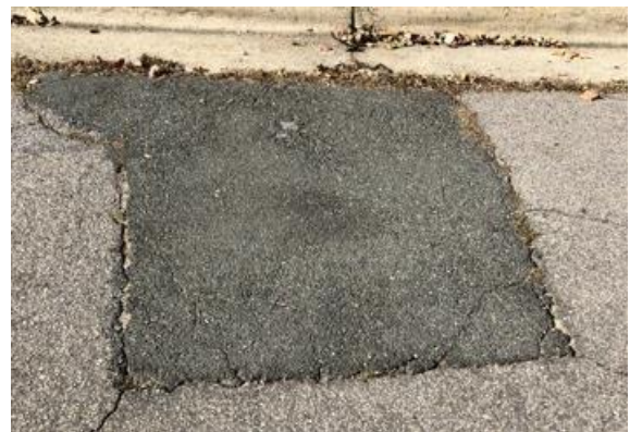
MEDIUM Severity Patch
