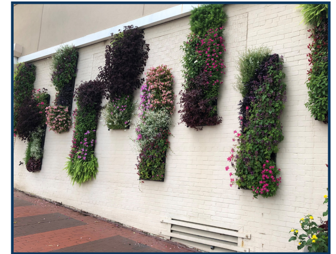
Use of living walls
