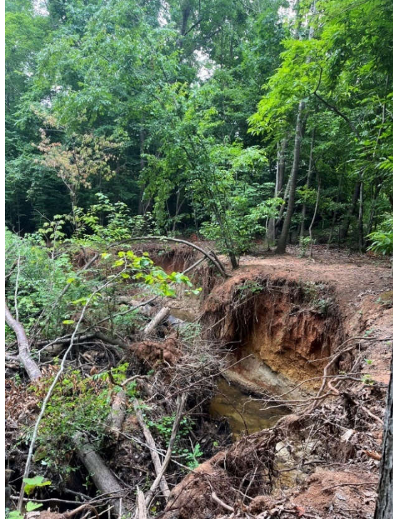
Area of eroded bank/lack of vegetation.
